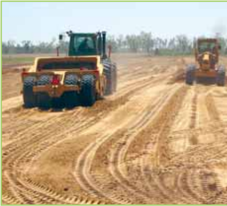
Fig. 1. Prior to the installation of the irrigation system, the topsoil was removed to a depth of 12" and stockpiled.
